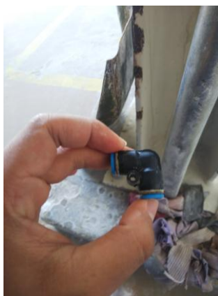
Gambar 2. 19 Elbow pipa pneumatik bocor
