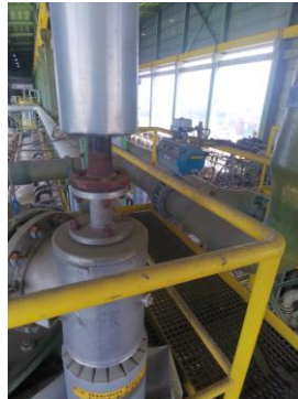
Gambar 2. 36 Temperature control valve evaporator
