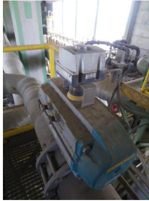
Gambar 2. 24 Temperature control valve
