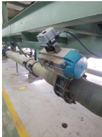
Gambar 2. 21 control valve spinbath evaporator
