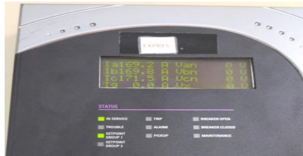
Gambar 2.57 Pengecekan beban feeder (Sumber: PT. Adra Gemilang 2022)
