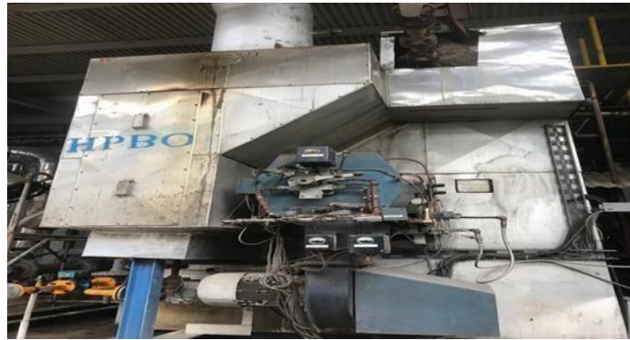
Gambar 2.4 High Preassure Boiler
