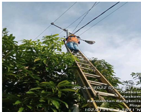
Gambar 2.16 Mengatasi Gangguan lost contact Nol/Netral (Sumber: PT. Adra Gemilang 2020)
