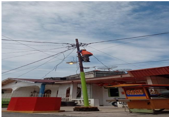
Gambar 2.33 Mengatasi Gangguan lost contact Nol/Netral (Sumber: PT. Adra Gemilang 2020)
