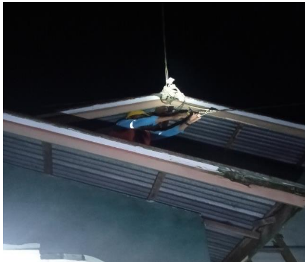
Gambar 2.45 Mengatasi Gangguan lost contact Nol/Netral (Sumber: PT. Adra Gemilang 2022)
