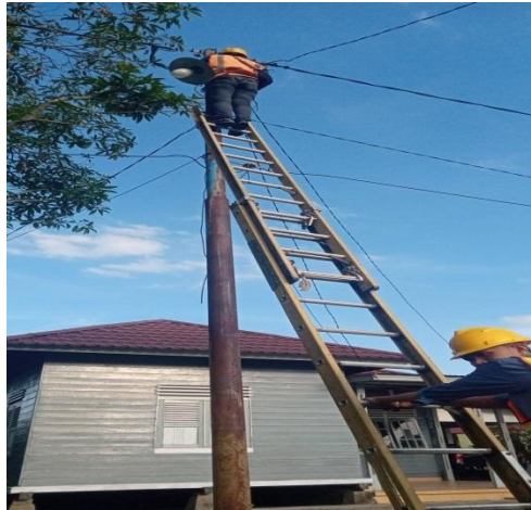
Gambar 2.22 Mengatasi Gangguan lost contact Nol/Netral (Sumber: PT. Adra Gemilang 2020)
