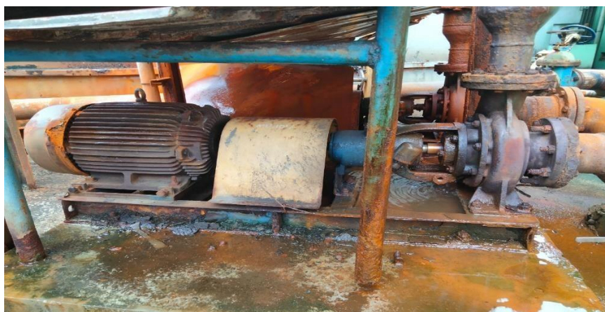
Gambar 4. 2 pompa sentrifugal pentransfer air
