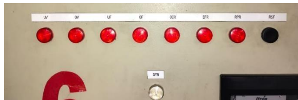
Gambar 3.13 Lampu Indikator Sinkron (Sumber: PT. Megapower Makmur Tbk. 2021)
