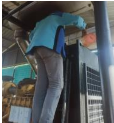
Gambar 2.21 Kegiatan penambahan air radiator (Sumber: PT. Megapower Makmur Tbk. 2022)
