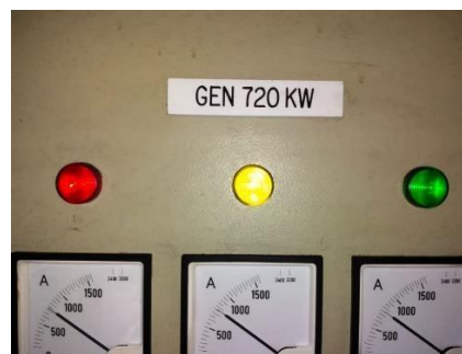
Gambar 3.4 Lampu Indikator Panel Sinkron (Sumber: PT. Megapower Makmur Tbk. 2021)
