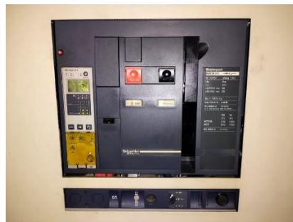
Gambar 3.14 ACB Panel Sinkron (Sumber: PT. Megapower Makmur Tbk. 2021)
