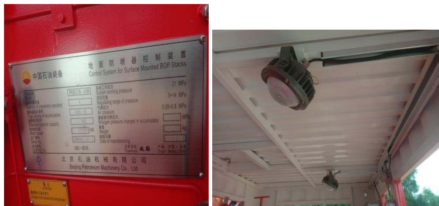
Gambar 2. 6 Pemasangan lampu outdoor atau lampu Merkuri di mesin Control System For Surface Mountes bop Stack . (Sumber: Dokumentasi,2022)
