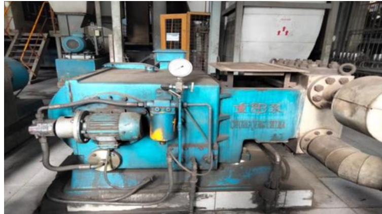
Gambar 4.1 Boiler feed water pump Sumber: PT. Wilmar Nabati Indonesia
