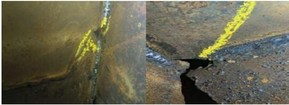
Gambar 2. 64 hasil visual Welding void tank H-594
