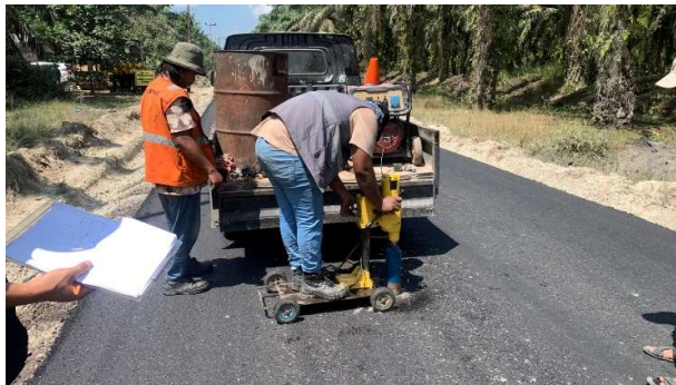
Gambar 3 32 pengujian Core Drill AC-BC
