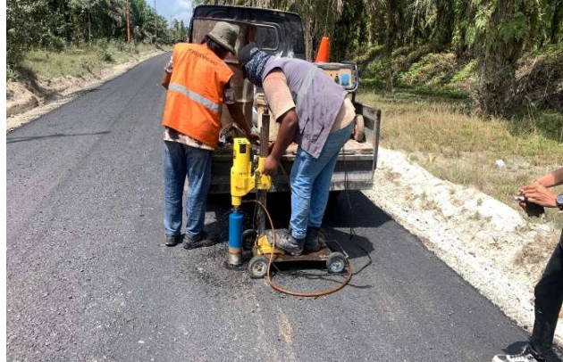
Gambar 4 12 Pengujian Core Drill AC BC
