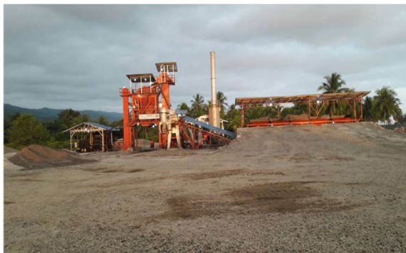
Gambar 3 12 Asphal Mechine Plant,PT BMA
