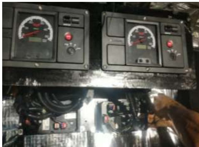
Gambar 2.8. 1 melihat instal kabel maen engine control
