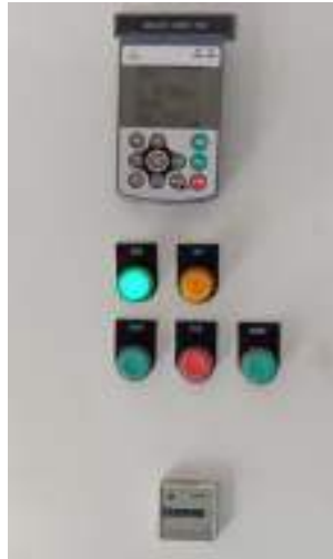
Gambar 4. 11 Pengukur ampere induced draught fan (Sumber : Dokumentasi 2025)
