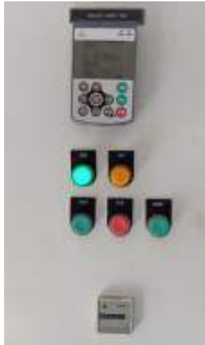
Gambar 4. 11 Pengukur ampere induced draught fan (Sumber : Dokumentasi 2025)
