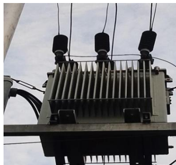
Gambar 4. 1 Transformator step-down Gardu Distribusi
