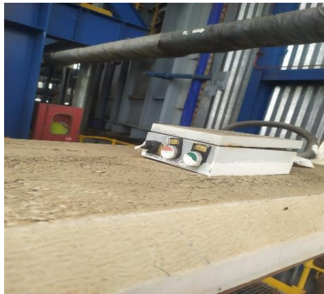
Gambar 4.10 Electrical Equipment (Sumber: Dokumentasi Pribadi)
