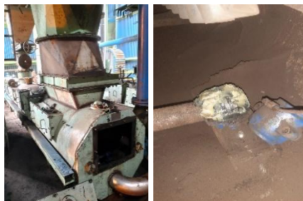
Gambar 3. 20 Coal Feeder (Sumber Dokumentasi: PT. Power Plant)
