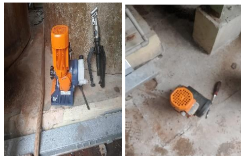
Gambar 3. 26 Motor pompa Housing (Sumber Dokumentasi: PT. Power Plant)
