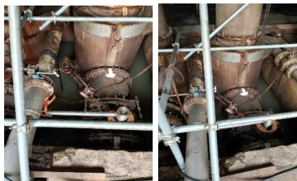
Gambar 3. 9 Close Manual Valve Inlet Kondensor Turbin2 (Sumber Dokumentasi: PT. Power Plant)
