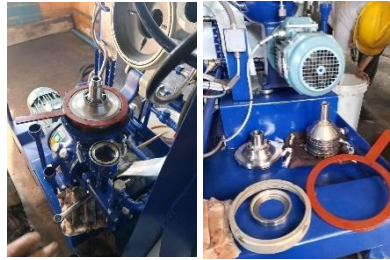
Gambar 3. 29 (Oil Cleaning Machine)-Purifier (Sumber Dokumentasi: PT. Power Plant)
