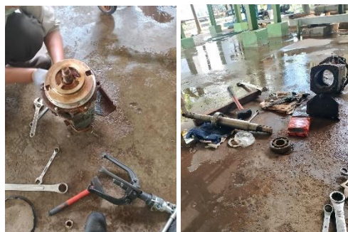
Gambar 3. 25 Pompa SWRO Feed2 (Sumber Dokumentasi: PT. Power Plant)
