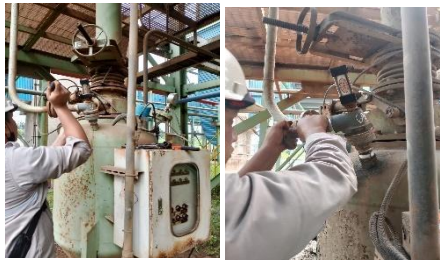
Gambar 3. 16 Air Lock Store Pump (Sumber Dokumentasi: PT. Power Plant)
