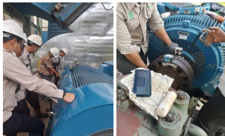
Gambar 3. 19 Alignment ID Fan (Sumber Dokumentasi: PT. Power Plant)
