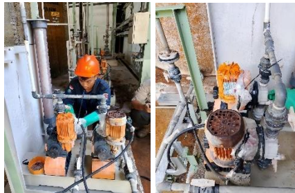
Gambar 3. 18 Pompa Hausing (Sumber Dokumentasi: PT. Power Plant)
