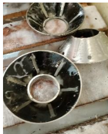
Gambar 4. 11 Sliding Bowl (Sumber Dokumentasi: PT. Power Plant)
