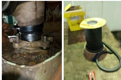
Gambar 3. 27 Motor pompa Housing (Sumber Dokumentasi: PT. Power Plant)
