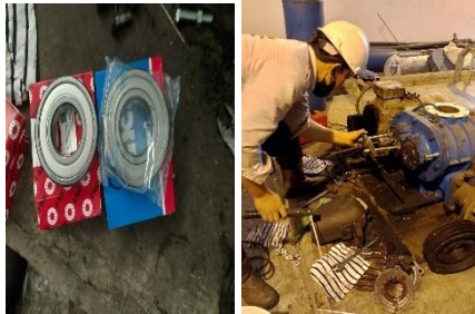
Gambar 3. 14 Bearing Pulley Air Blower K001 (Sumber Dokumentasi: PT. Power Plant)
