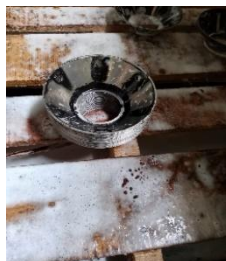
Gambar 4. 5 Disk Stack (Sumber Dokumentasi: PT. Power Plant)
