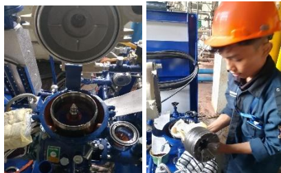
Gambar 3. 15 OCM (Oil Cleaning Machine)-Purifier (Sumber Dokumentasi,PT. Power Plant)
