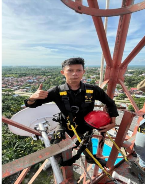
Gambar 3. 11 Penanganan Gangguan Radio Di Tower Central Surya
