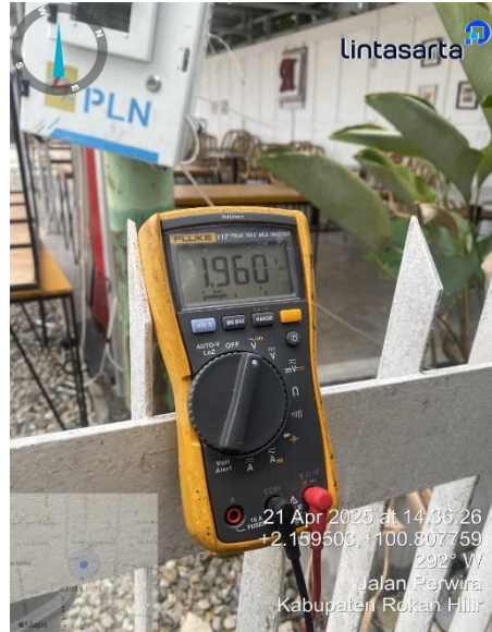
Gambar 3. 17 Preventive maintenance cek watt listrik
