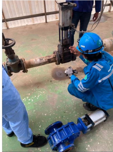
Gambar 2. 7 Penggantian Pneumatic Valve
