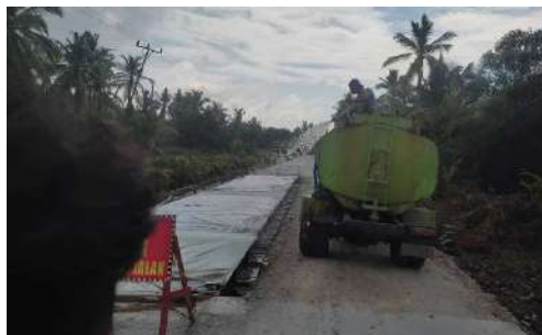
Gambar 4.4 Water Tank Truck Sumber :Dokumentasi Lapangan 2024
