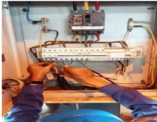
Gambar 3. 25 support power Sumppump
