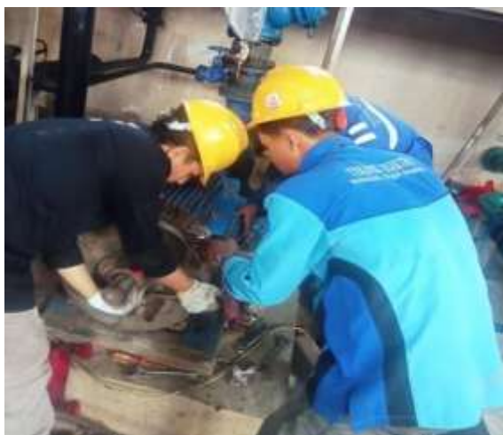
Gambar 3. 100 Gambar PAM area WTP
