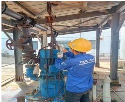
Gambar 3. 77 connect power motor Wash Water Pump A
