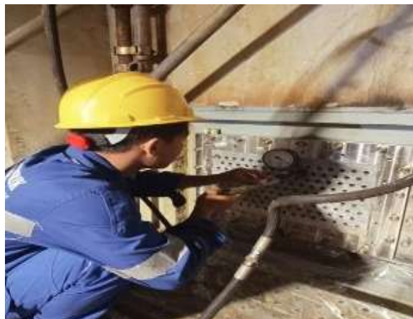
Gambar 3. 64 vacuum test cooler generator unit 2
