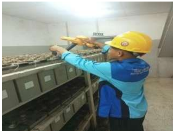
Gambar 3. 37 preventive maintenance batere eksitatsi
