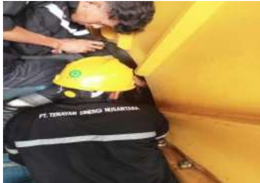
Gambar 3. 83 Preventive Maintenance generator
