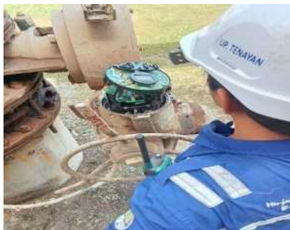
Gambar 3. 49 penormalan dan pengecekan MOV area Cooling tower unit
