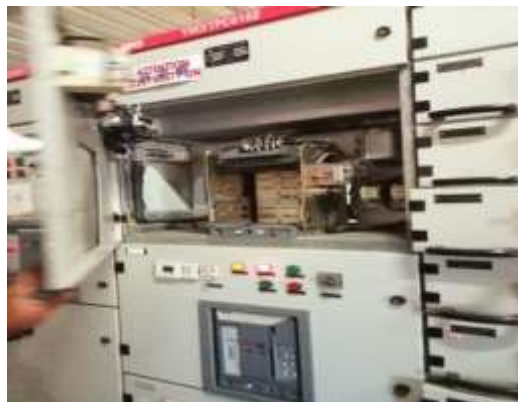
Gambar 3. 76 connect power motor Wash Water Pump A
