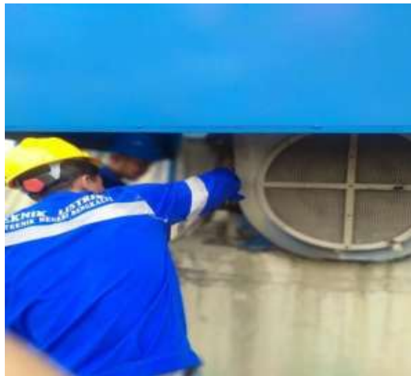
Gambar 3. 93 Gambar motor cooling tower
