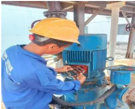
Gambar 3. 75 connect power motor Wash Water Pump A
