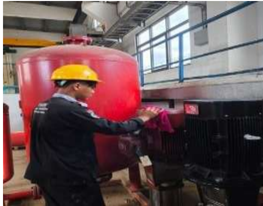
Gambar 3. 79 preventive maintenance motor industrial
