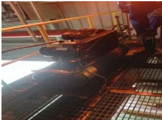
Gambar 3. 42 mobilitasy compresor Bus Duct Unit
