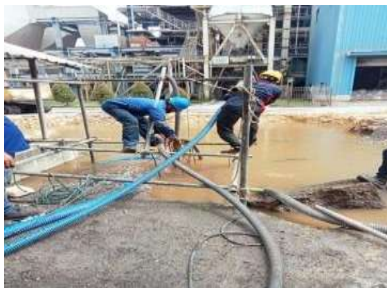
Gambar 3. 43 support connect power sumppump 3 fase
