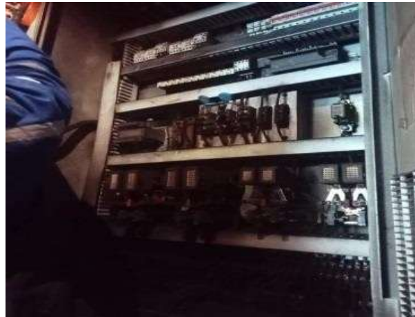
Gambar 3. 20 pengecekan panel magnetic separator C03
