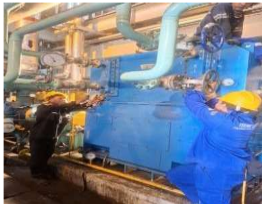
Gambar 3. 84 Preventive Maintenance generator
