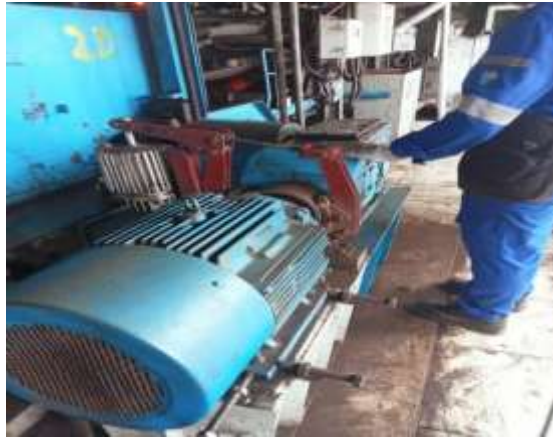
Gambar 3. 44 preventive maintenance motor
