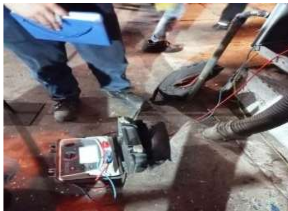
Gambar 3. 54 Magger Motor Boiler Feed Pump
