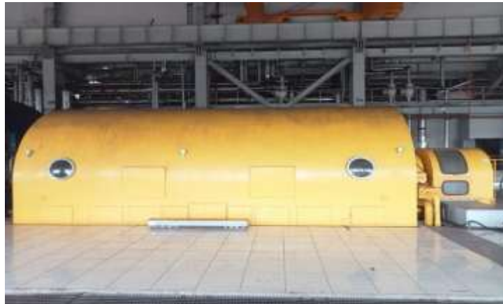
Gambar 4. 1 Generator PLTU Tenayan
