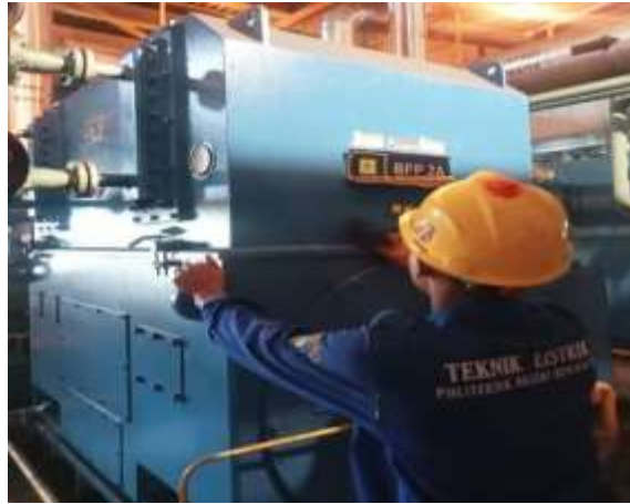
Gambar 3. 96 PM Motor Boiler feed pump
