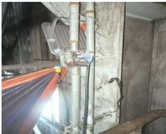
Gambar 3. 41 support power Outlet CF2D
