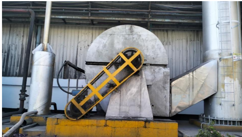
Gambar 4. 4: Induced Draft Fan (ID FAN) Sumber : PT.pacific indopalm industries
