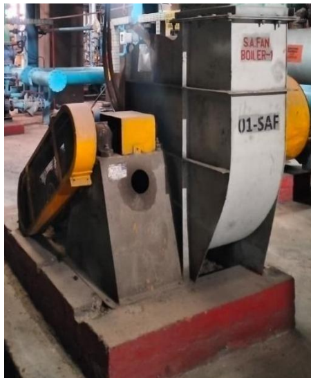
Gambar 4. 5: Secondary Air Fan (SA FAN) Sumber : PT. pacific indopalm industries
