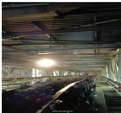
Gambar 4. 1 gambar conveyor (Sumber : Dokumentasi PT. Power Plant )
