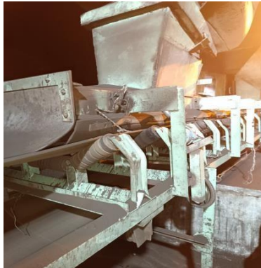
Gambar 4. 10 Discharge Chute (Sumber : Dokumentasi PT. Power Plant)
