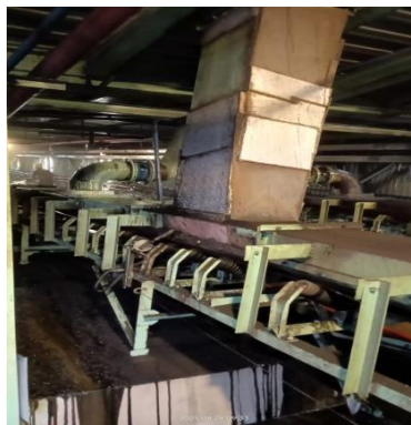
Gambar 4. 9 Loading Chute (Sumber : Dokumentasi PT. Power Plant )
