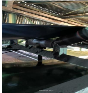
Gambar 4. 4 Idler Roller (Sumber : Dokumentasi PT. Power Plant )
