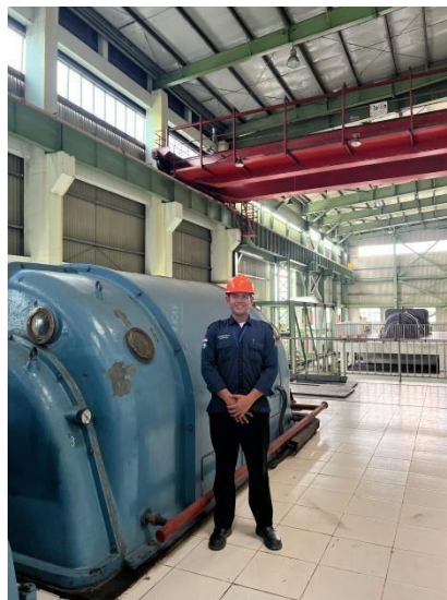
Gambar 4. 1 turbine (Sumber : Dokumentasi PT Power Plant )
