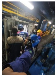
Gambar 3. 28 MCC Preheater Fault
