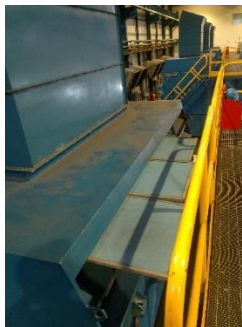
Gambar 3. 47 Filter Udara generator
