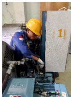
Gambar 3. 21 Motor compressor starting
