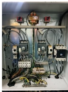
Gambar 3. 29 Panel Kontrol Compressor
