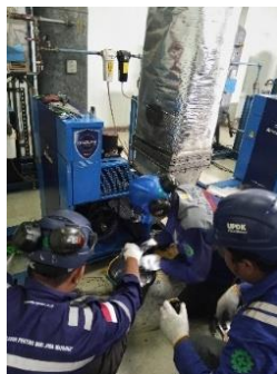
Gambar 3. 41 Compresor Instrumen Air
