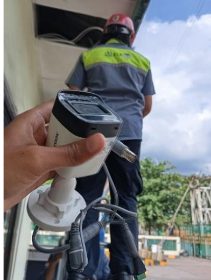
Gambar 3. 7 Instal Unit CCTV Di PT KJA
