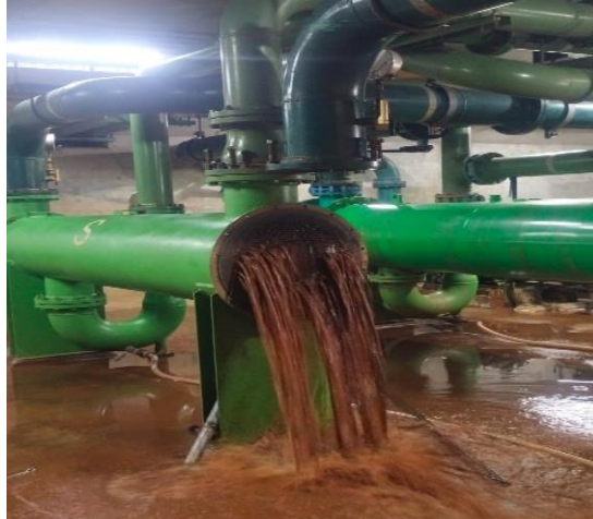
Gambar 3.89 Pencucian HE(Heat exchanger)
