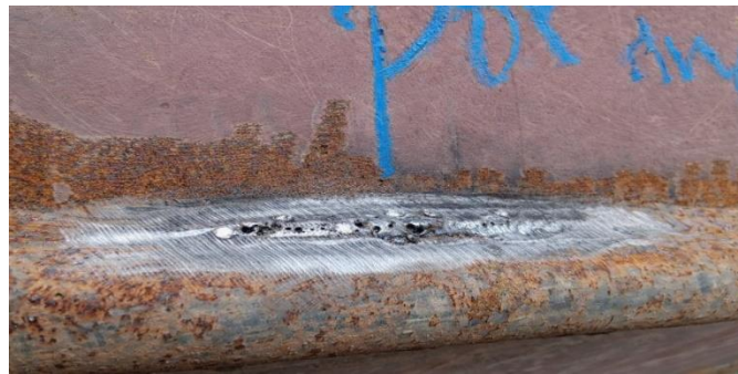
Gambar 4.1 Porosity welding defect before full grinding
