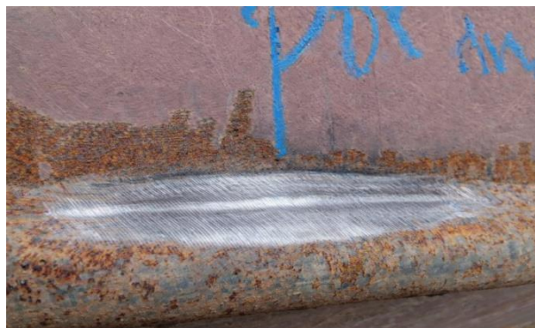
Gambar 4.2 Porosity welding defect after full grinding
