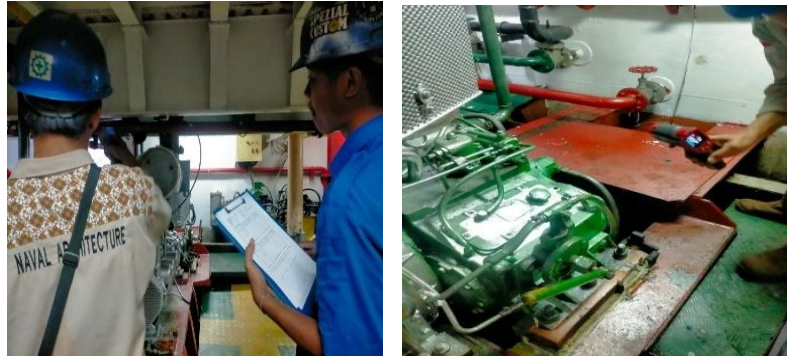
Gambar .3.61 dock trail KMP JAMBO VI
