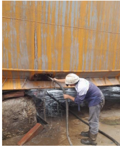
Gambar 3.27 Hose test TB.HARLINA 3
