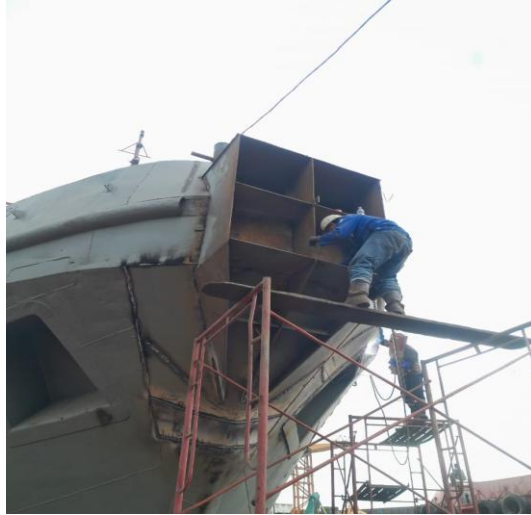
Gambar 3.33 Penetrant test TB.HARLINA 3
