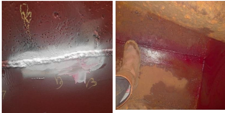
Gambar 3.39 Penetrant Test TB.HARLINA 3
