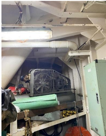
Gambar 3. 60 Tampak mesin compressor
