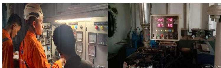
Gambar 3. 47 Load Bank Generator
