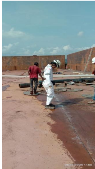
Gambar 3. 23 External air Pressure Test Tank
