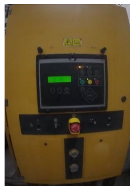
Gambar 4. 7 panel control genset sumber pt esm
