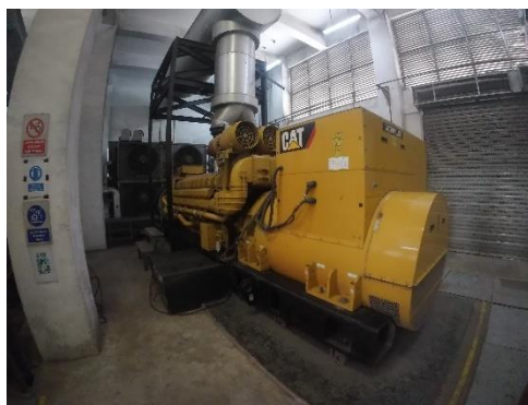
Gambar 4. 3 Genset open type sumber PT. ESM
