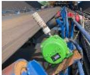
Gambar 3.13 Sensor Belt Sway Sumber: PT.PLN Nusantara Power
