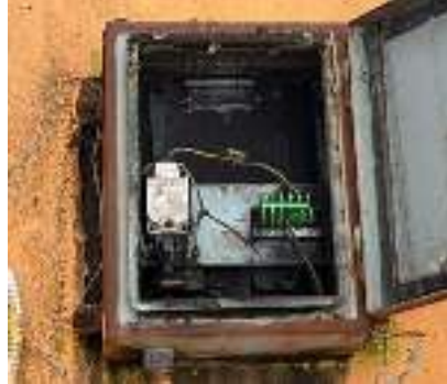
Gambar 3. 14 Sensor Blocket Sumber: PT.PLN Nusantara Power
