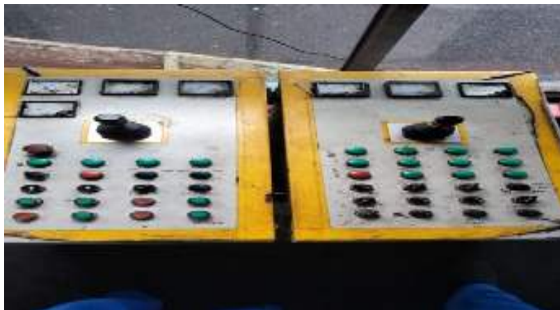
Gambar 3. 10 Control PLC Sumber: PT.PLN Nusantra Power
