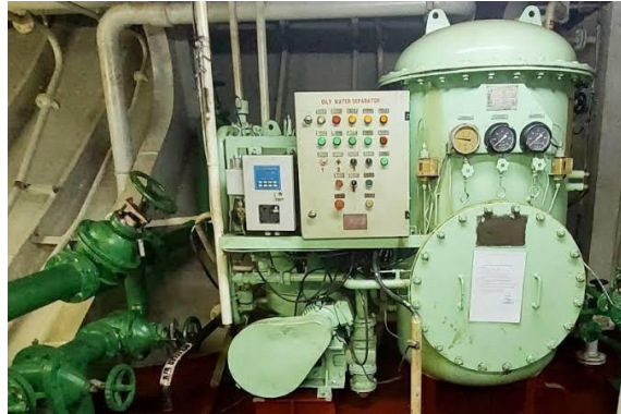
Gambar 2. 6 Oil Water Separator
